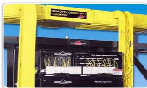
Fiber Cable Raceway
