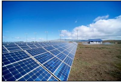
Figure 39: Solar panel system
