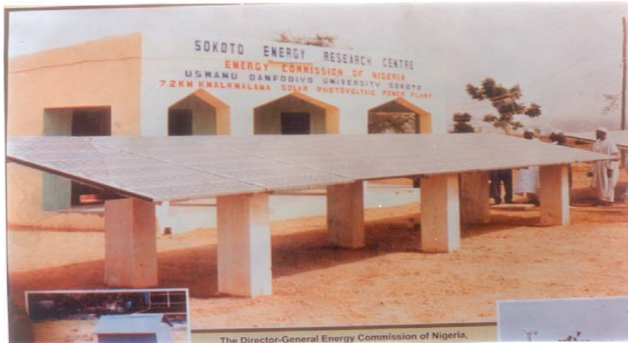
Fig. 14. 7.2 kWp Village Electrification, Kwalhwalawa, Sokoto State
