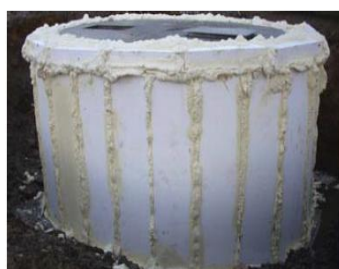
Tank 2 with a total of 600mm insulation
