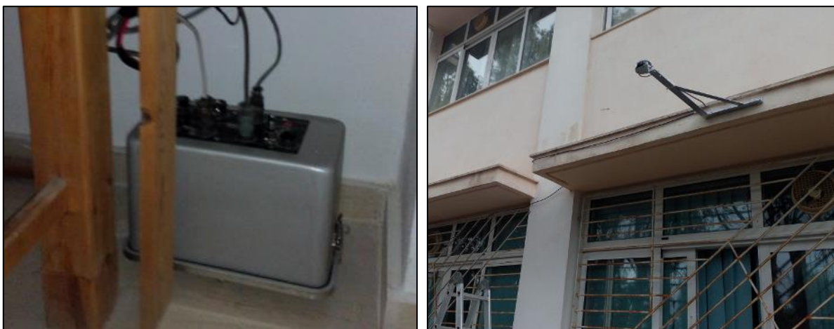
Figure 2.8 The GOLD SGM station, the installed REF TEK 130-SM (left)and the external GPS antenna(right).
