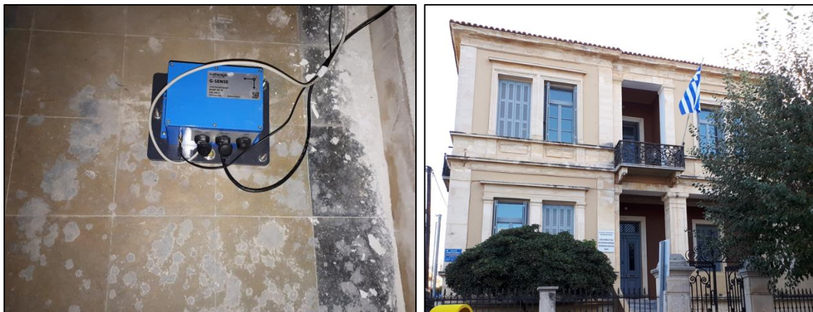
Figure 2.6 The GSense sensor (left) of the ATIK SGM station in the Neoclassic building (right).
